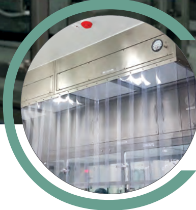
AIR FLOW UNIT
